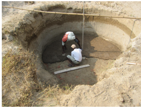
Concreting the base for the new Bio Gas Oven at Punarnawa Ashram – 23 November 2010
