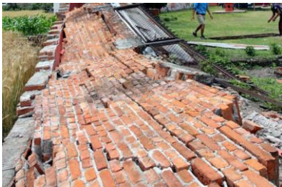
Maiti Hospice wall after the April 2015 earthquake
